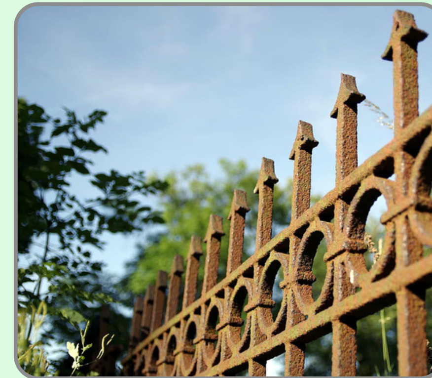
Corrosion of iron railings
