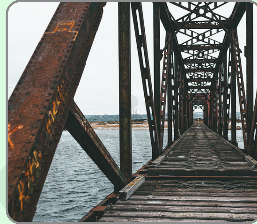
Corrosion on bridges
